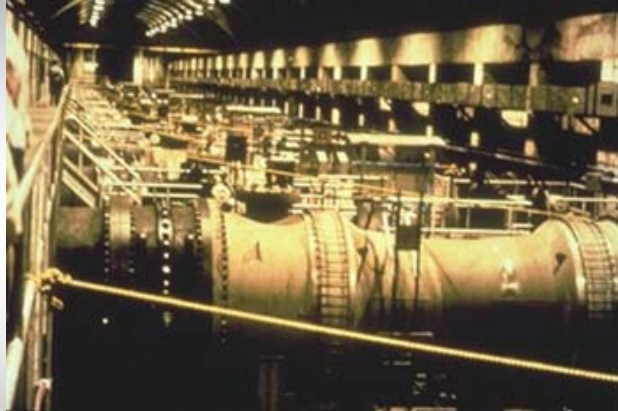
One of 3 pumping stations using cast stainless steel laterals and wrought butterfly valves
