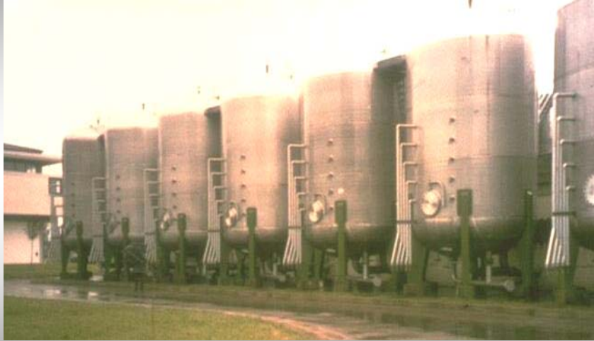
316L granular activated carbon tanks, Italy
