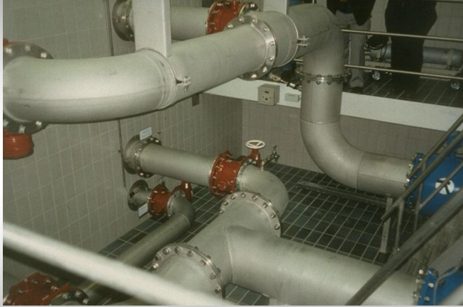
316Ti pipework in Germany
