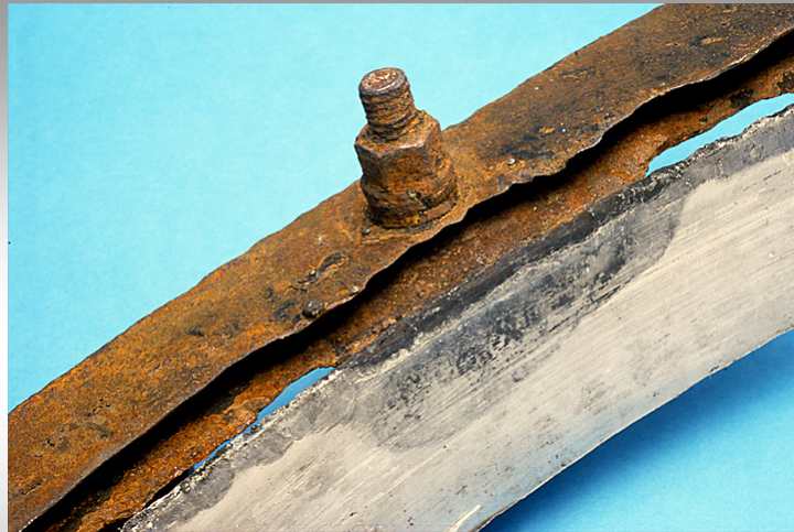
Galvanic corrosion between a carbon steel support ring and the large Type 304 hot water storage tank to which is was welded. The tank was lagged with fibreglass and water leaked into the lagging.
