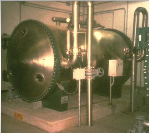
316 for ozone generator, Italy
