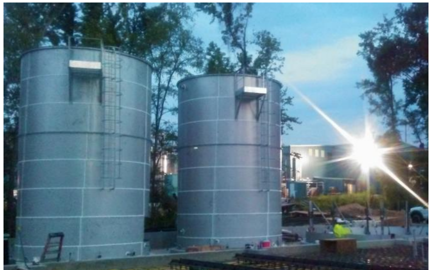
Zschimmer & Schwarz— Milledgeville, GA (3 tanks) 2— 18.46' x 28.83' EQ Tanks (57,718 gal. storage capacity) 1— 36.93' x 28.83' Aeration Tank (230,940 gal. storage capacity)
